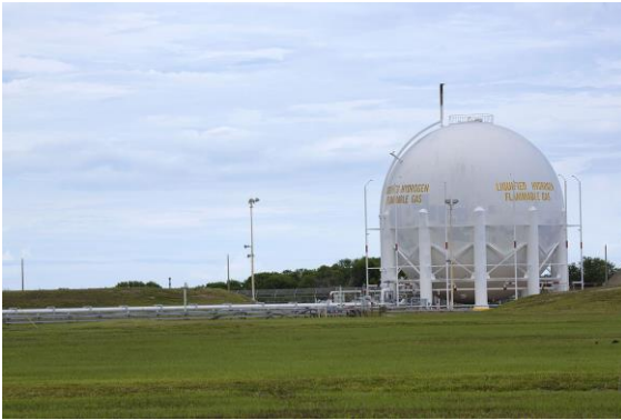
Liquid hydrogen storage tank
